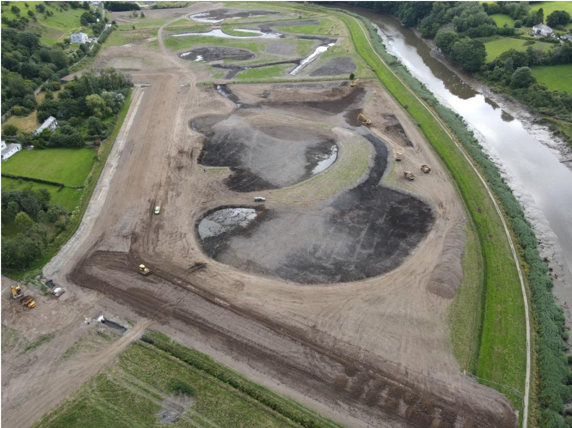
Flood embankments and habitat channels under construction. This area will become a reedbed habitat following the breach of the former flood embankment.
